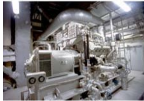
(Private power generator)
